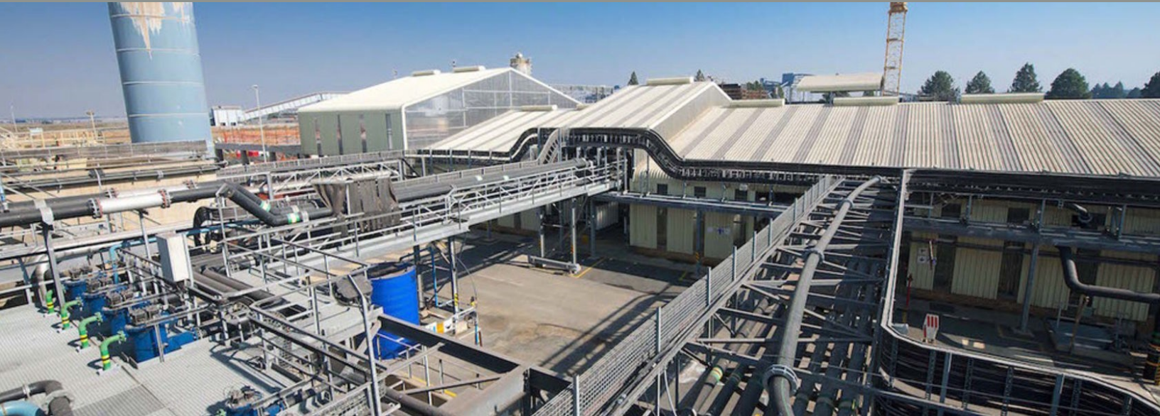
The eMalahleni water plant in South Africa
